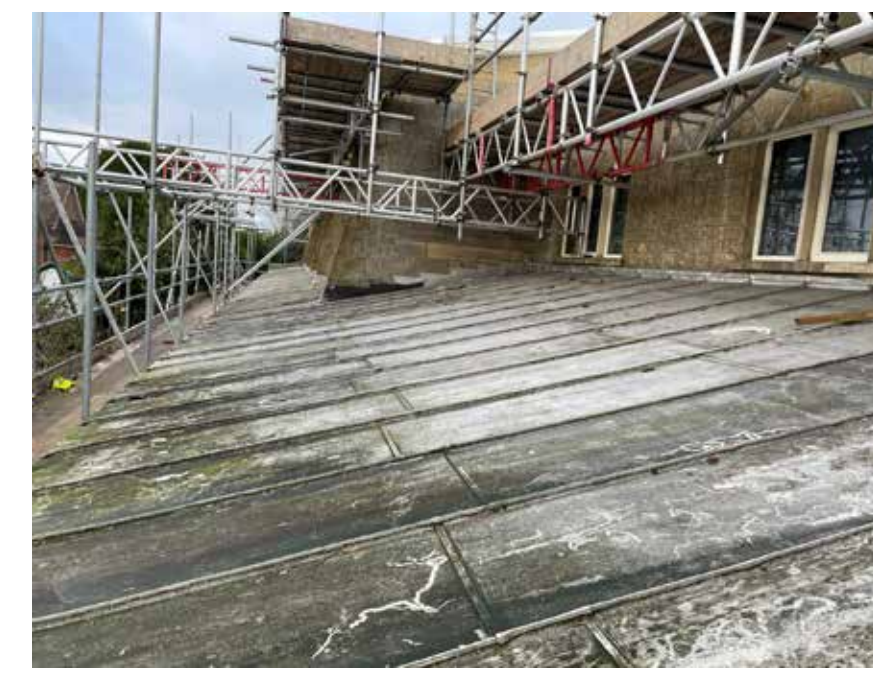
Close-up view of the existing roofs' surface highlighting the degradation.
