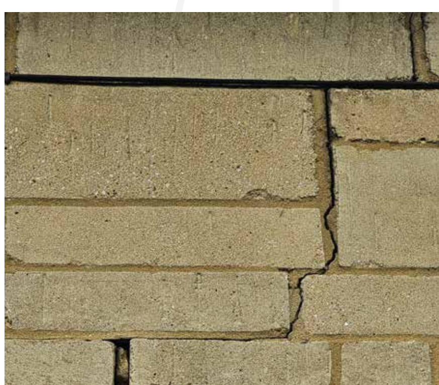
Extensive cracks to masonry evident.
